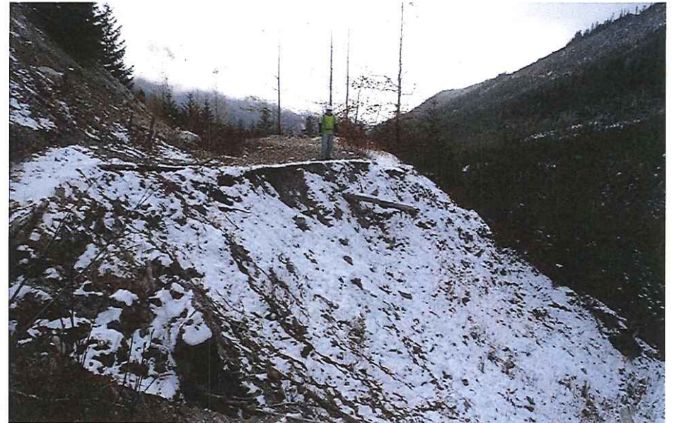
CK2205 Impassable road failure
